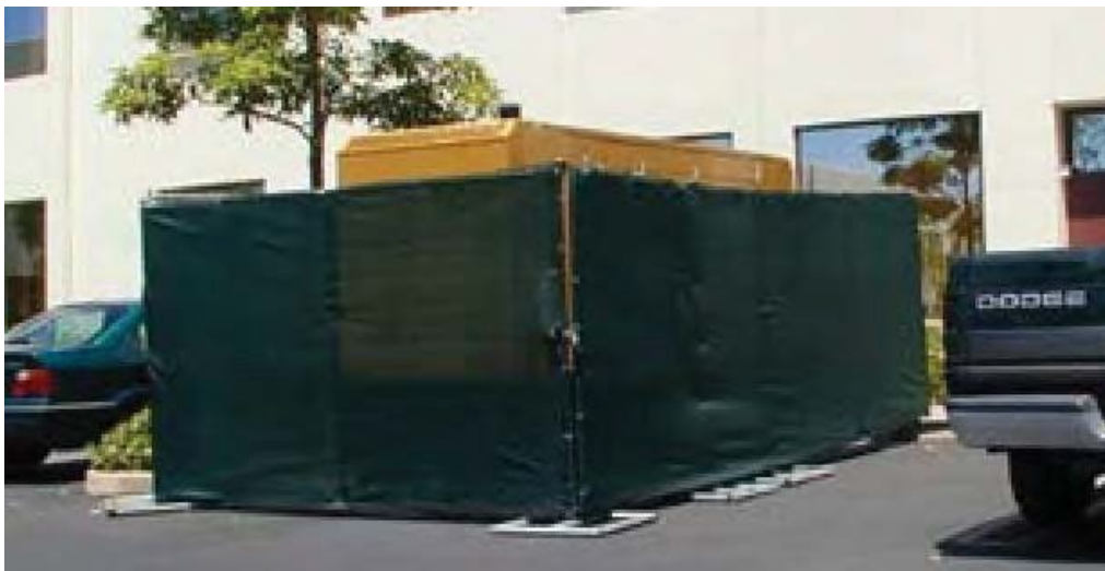
Figure 5-26 Example of Inappropriate Ground Mounted Equipment Screening
